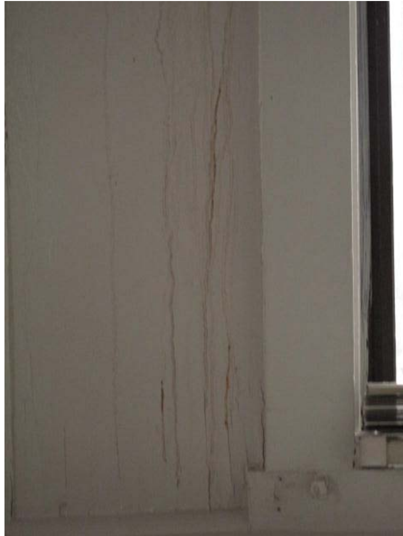
Moisture Damaged Walls
