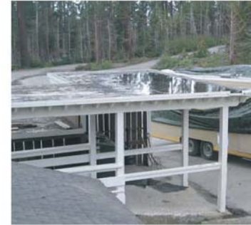
B3010-12: Roof B2 with standing water.
