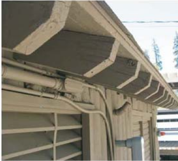
B3010-10: Deteriorated rafter tails.
