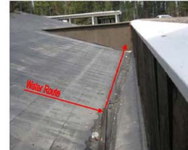
B3010-06: Water route at north retaining wall.
