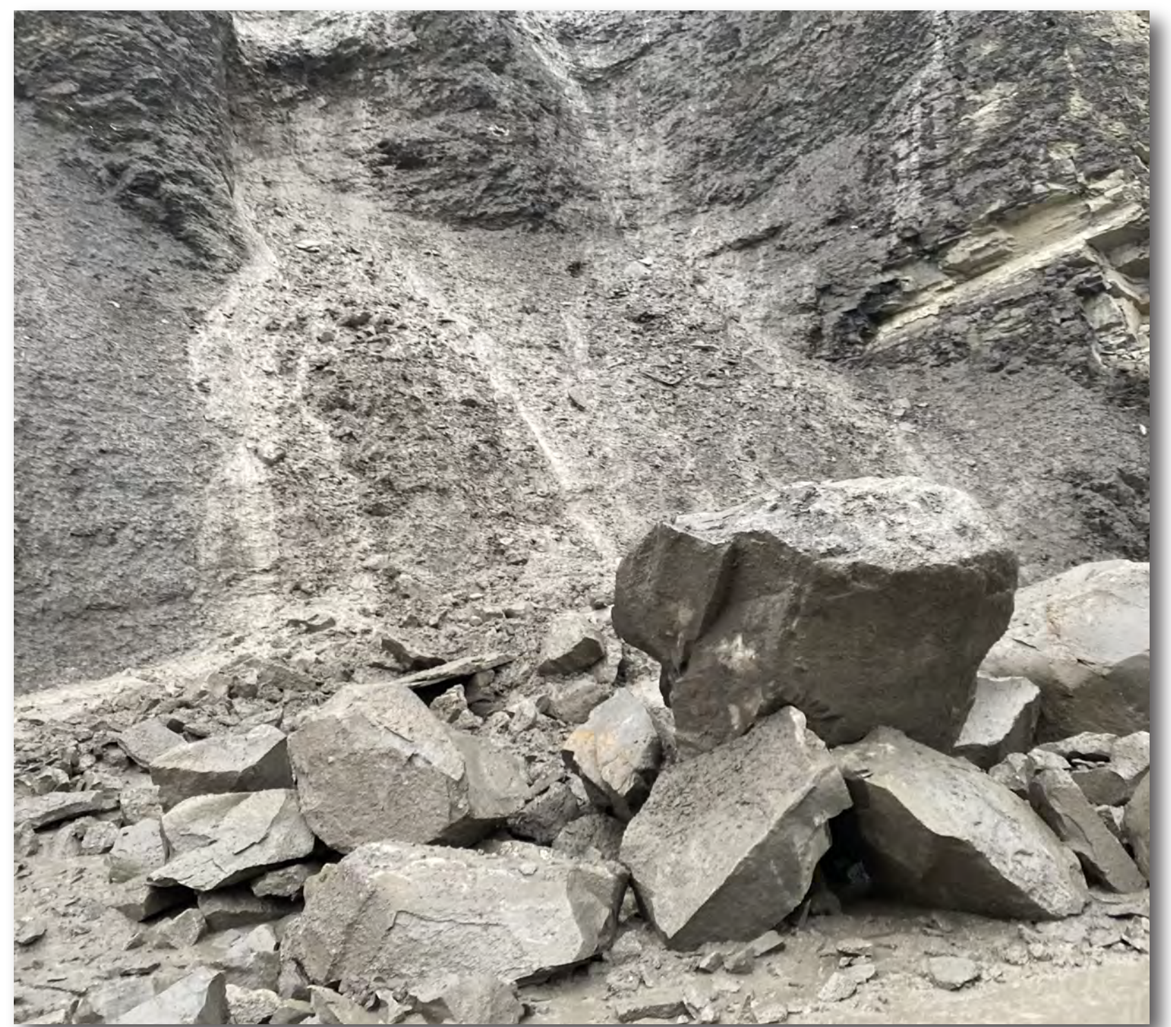
Large rockslide on North Entrance Road in the Gardner River Canyon. Retaining walls would be constructed to minimize geologic hazards and potential impacts on resources.
