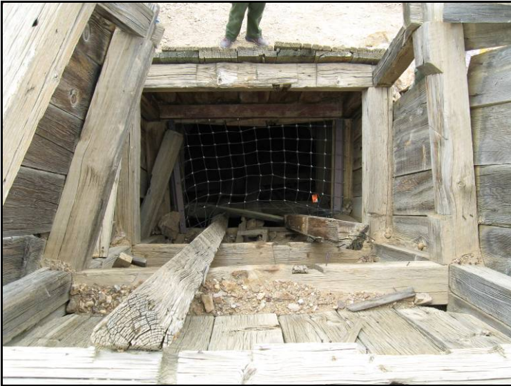
Photo 17. Net closure recessed in mine shaft.
