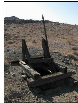
Photo 16. Shaft closed with a recessed bat gate. Note undisturbed area surrounding opening.
