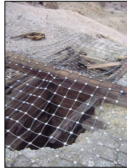
Photo 18. Cable net mine closure on a mine shaft.
