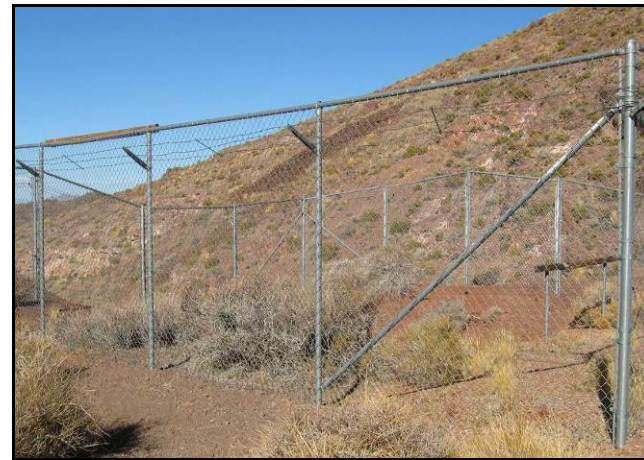
Photo 8. Fenced mine shaft closure incorporating wooden owl perches on top of the fence (left) and at the edge of the shaft (right)..
