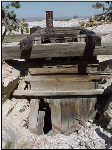
Photo 21. Unclosed vertical shaft conditions.
