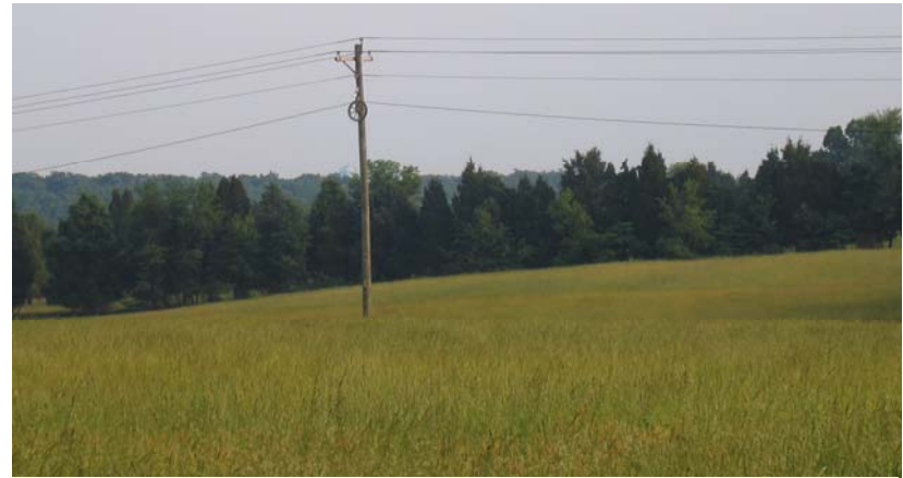
This type of conventional utility pole and overhead wiring exist throughout the battlefield area along roadways.
