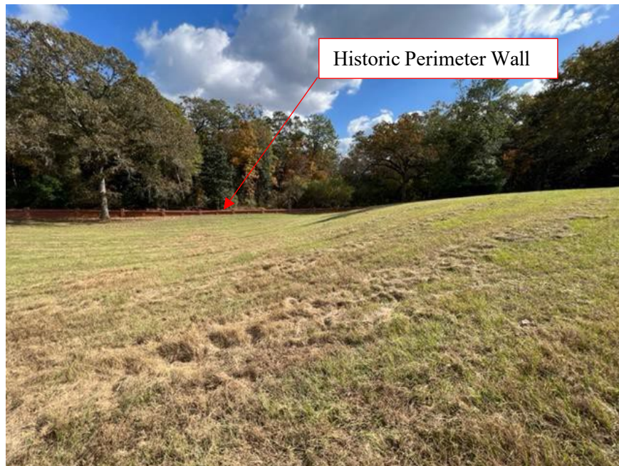
4b: Photo looking southeast across Section Q. Note the sloping drain running primarily from west to east down toward the historic cemetery perimeter brick wall.
