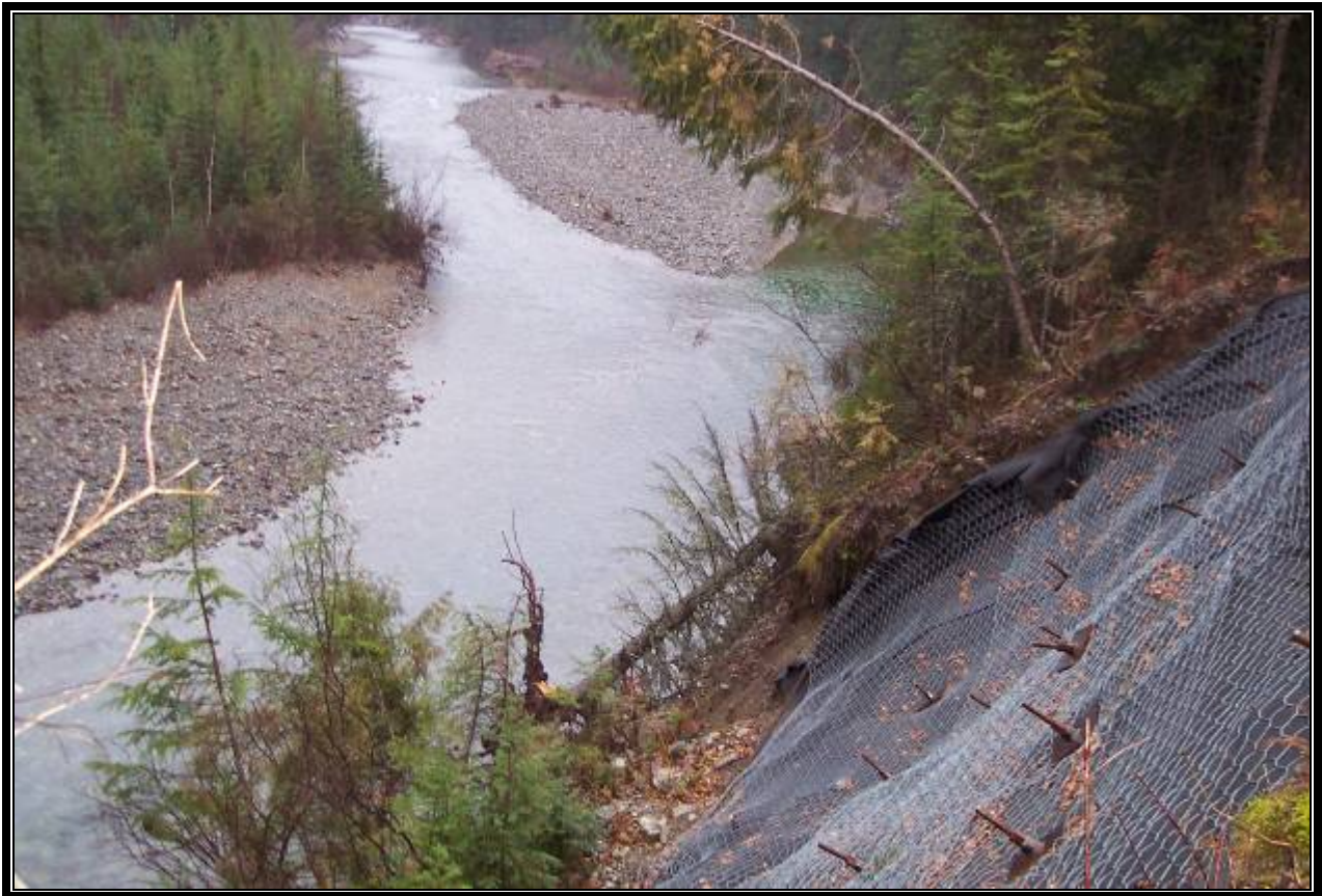
Slumping of shoulder at MP 19.25, November 2007
