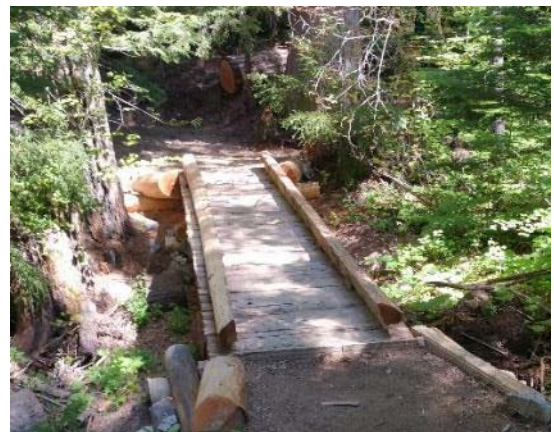
Figure 5. An example of a recently built puncheon bridge on the Thunder Creek Trail.
