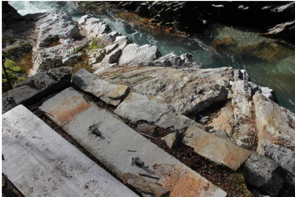
Figure 4. The bridge abutment in the foreground and Thunder Creek in a small gorge in the background where the bridge was washed out during the flood in late November 2017. Note the bent over bolts on the abutment.
