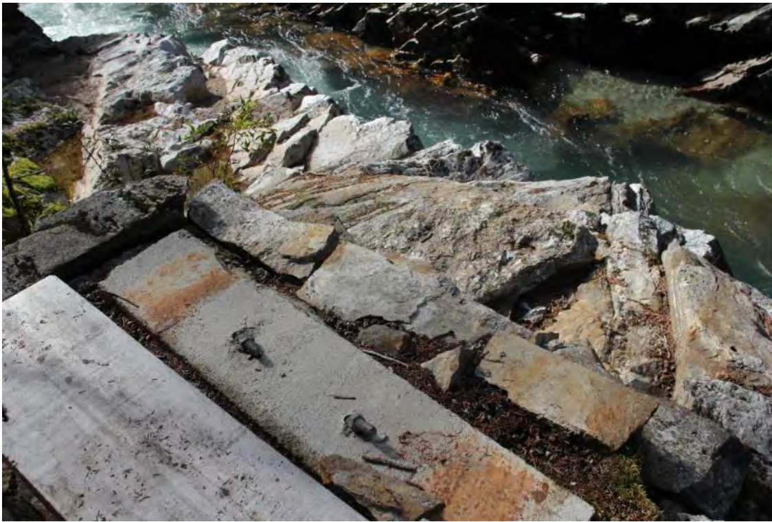
Figure 3. The bridge abutment in the foreground and Thunder Creek in a small gorge in the background where the bridge was washed out during the flood in late November 2017. Note the bent over bolts on the abutment.
