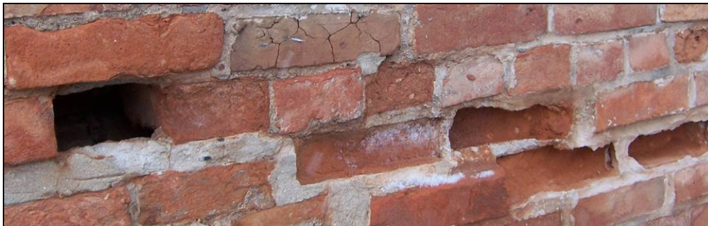
Figure 7: Deteriorating Chapel Bricks
