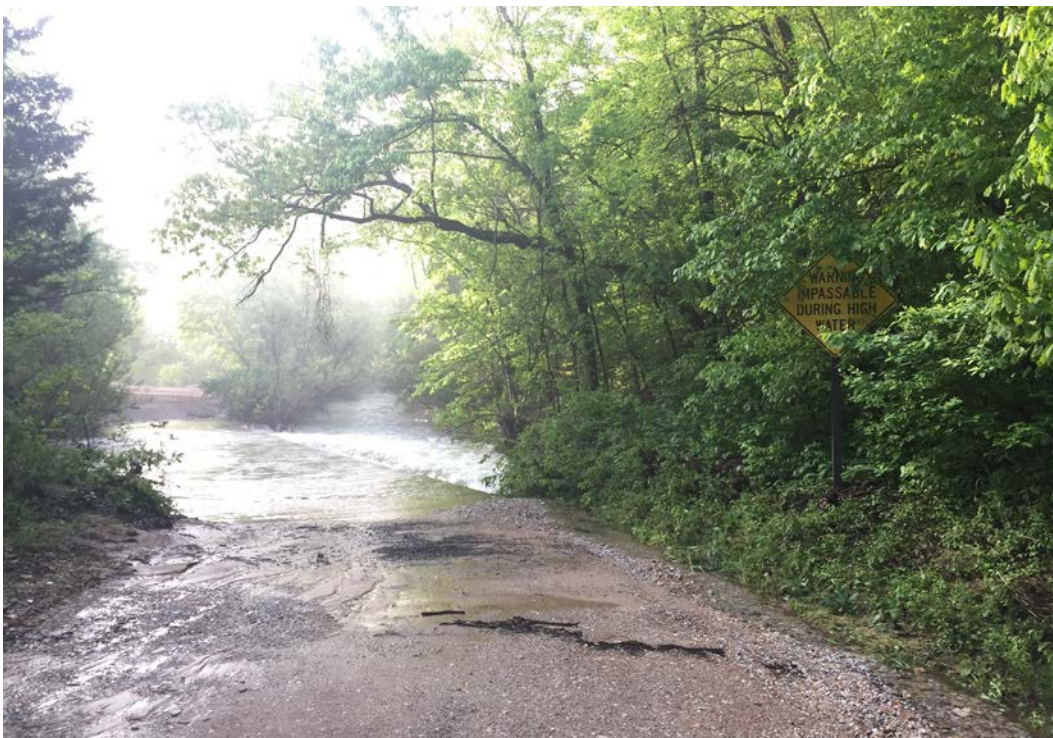
Figure 3-20. Rush Road crosses Rush Creek via a concrete water crossing near House Row. (Mundus Bishop 2017)
