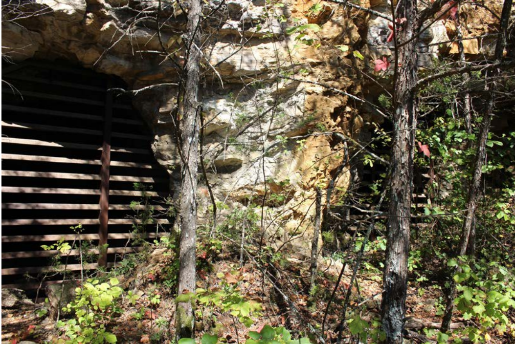
Figure 3-37. The lower entrances to McIntosh Mine (M5) are closed off with metal grates, typical of most horizontal mine portals. The dense vegetation makes it difficult to see the mine portals and rock face. (Mundus Bishop 2017)
