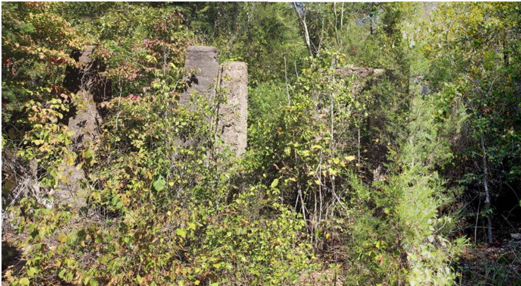
Figure 3-123. Morning Star Mill retention basin concrete spillway, same view as above. (Mundus Bishop 2017)
