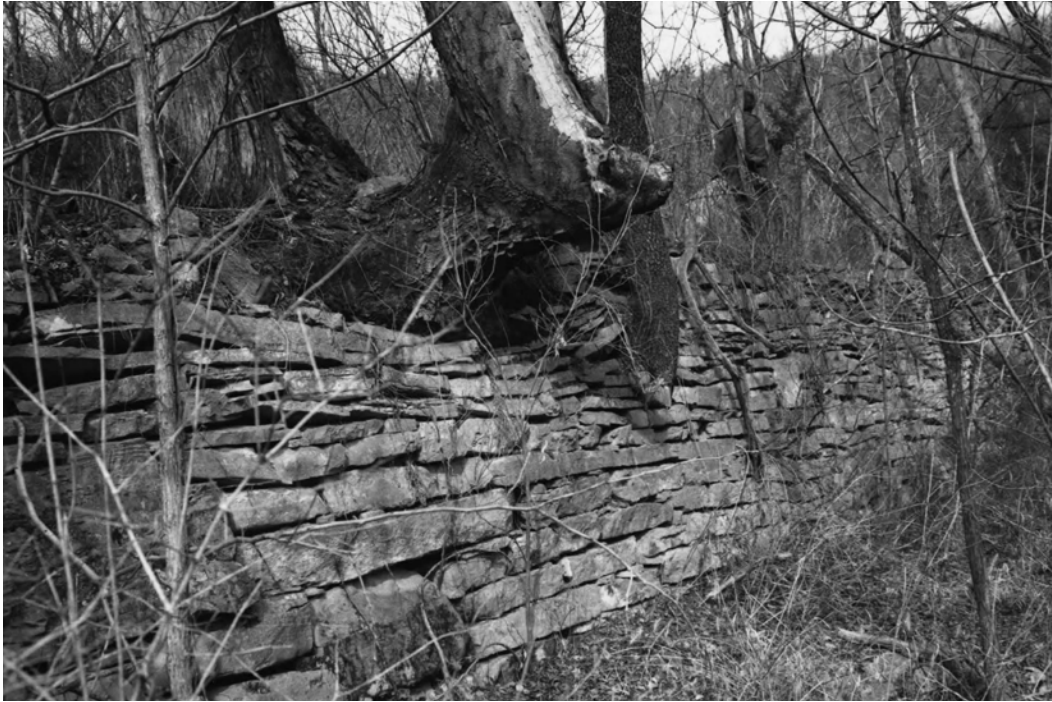
Figure 3-114. Portion of retaining wall at Morning Star Mill ruins, 1984. (S. Rogers, BUFF Archives)
