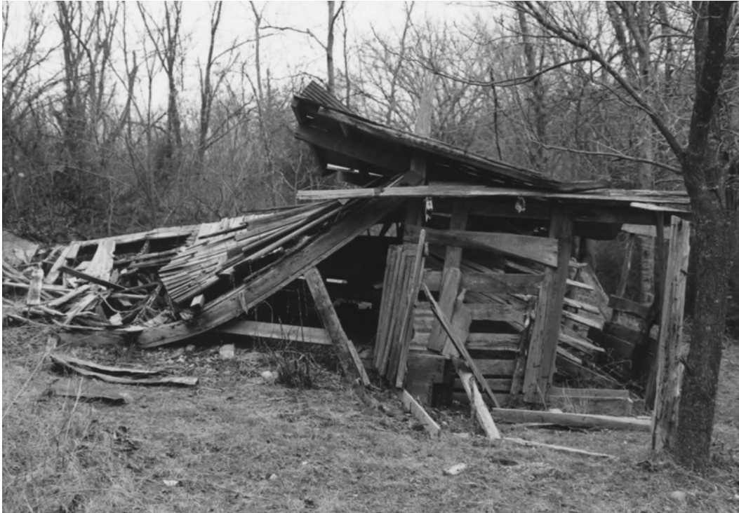
Figure 3-144. Collapsed Raby House, 1984. (S. Rogers, BUFF Archives)
