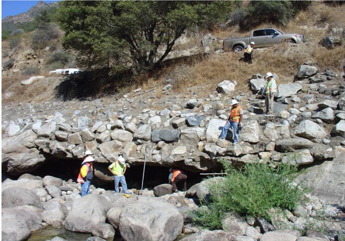
Photo 2 View of highway embankment showing the eroded void and vehicles on the highway shoulder.
