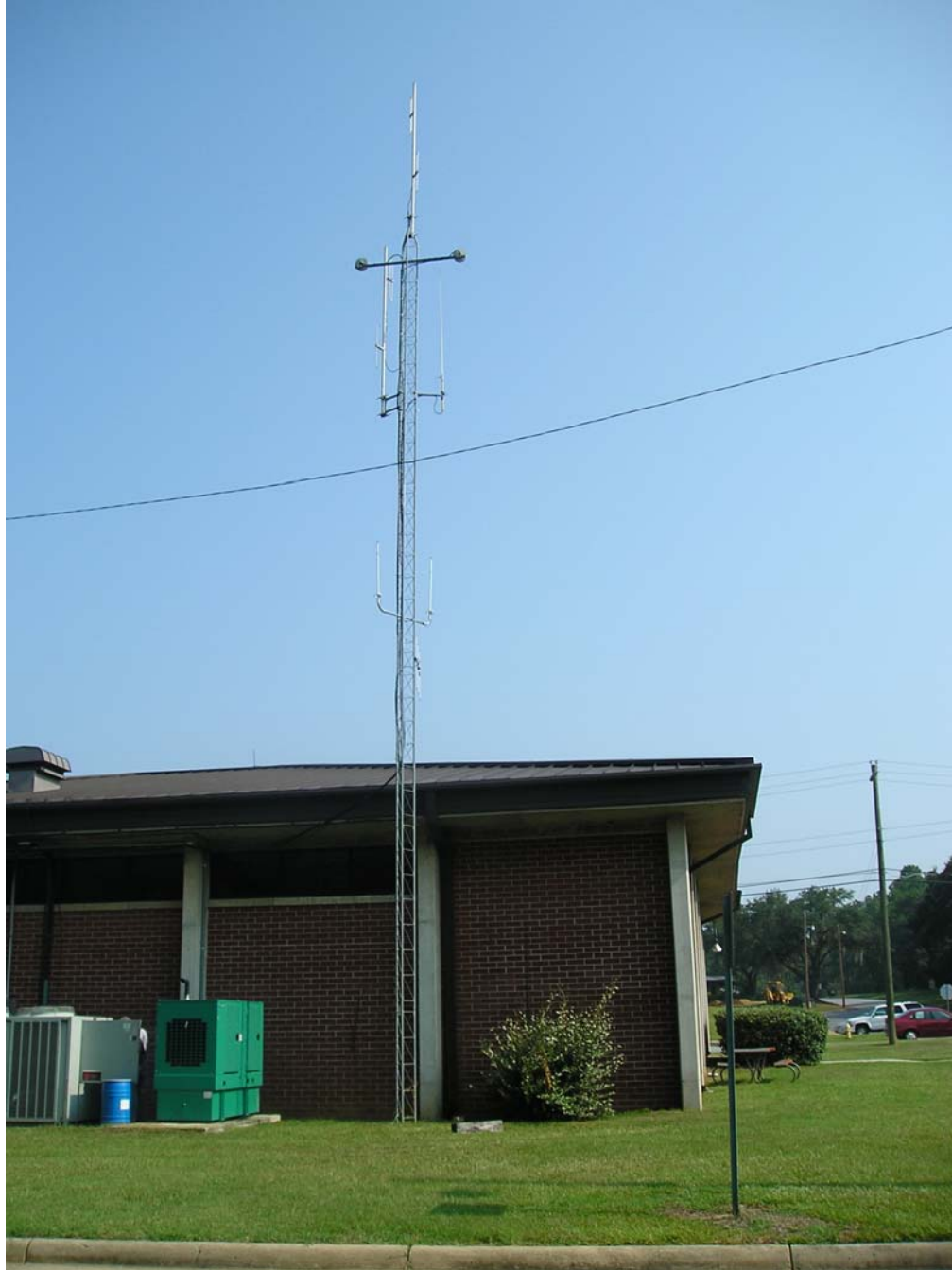
Example of a 60ft Self-Supporting Tower
