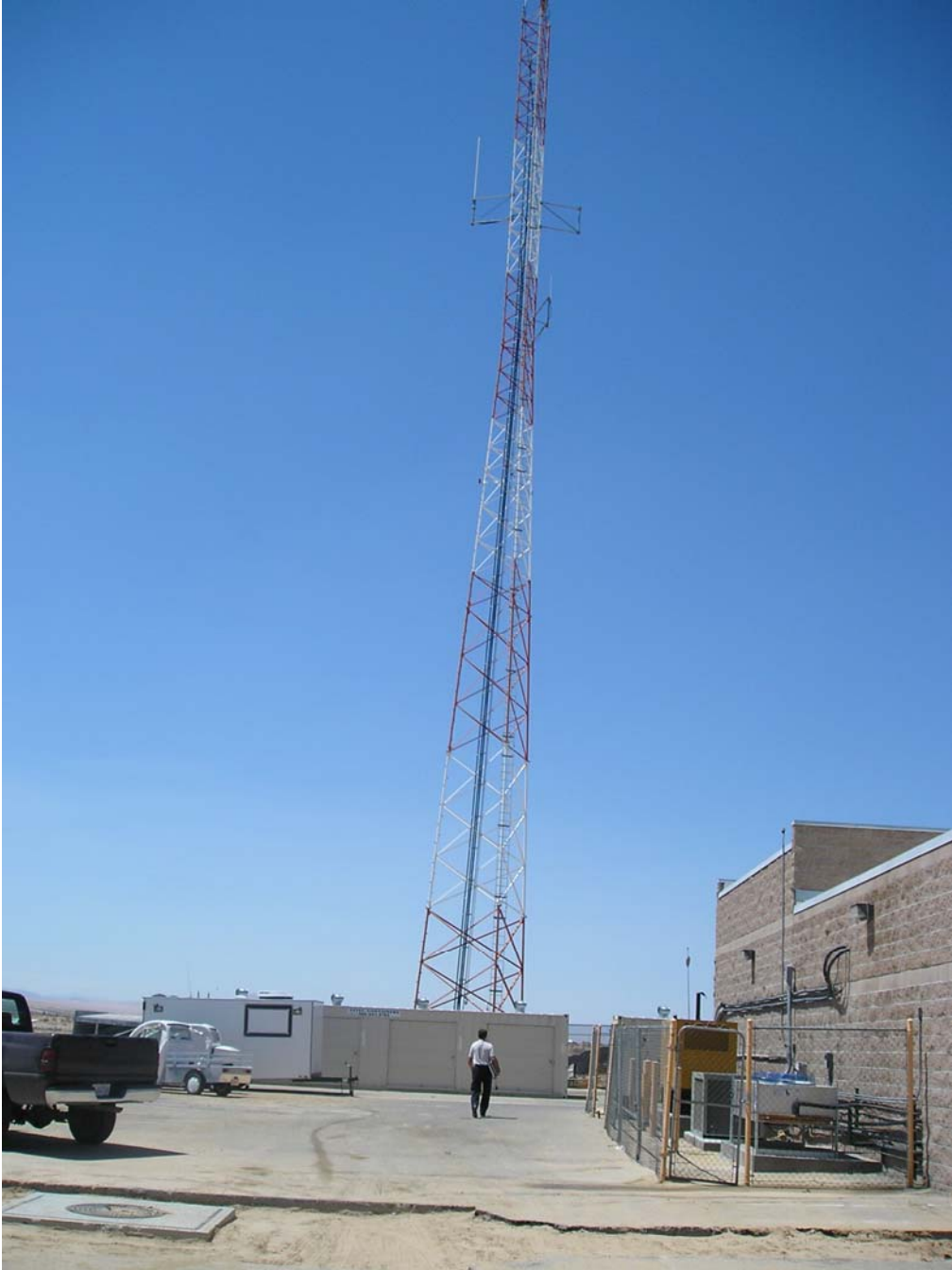
Example of a 100ft Self-Supporting Tower
