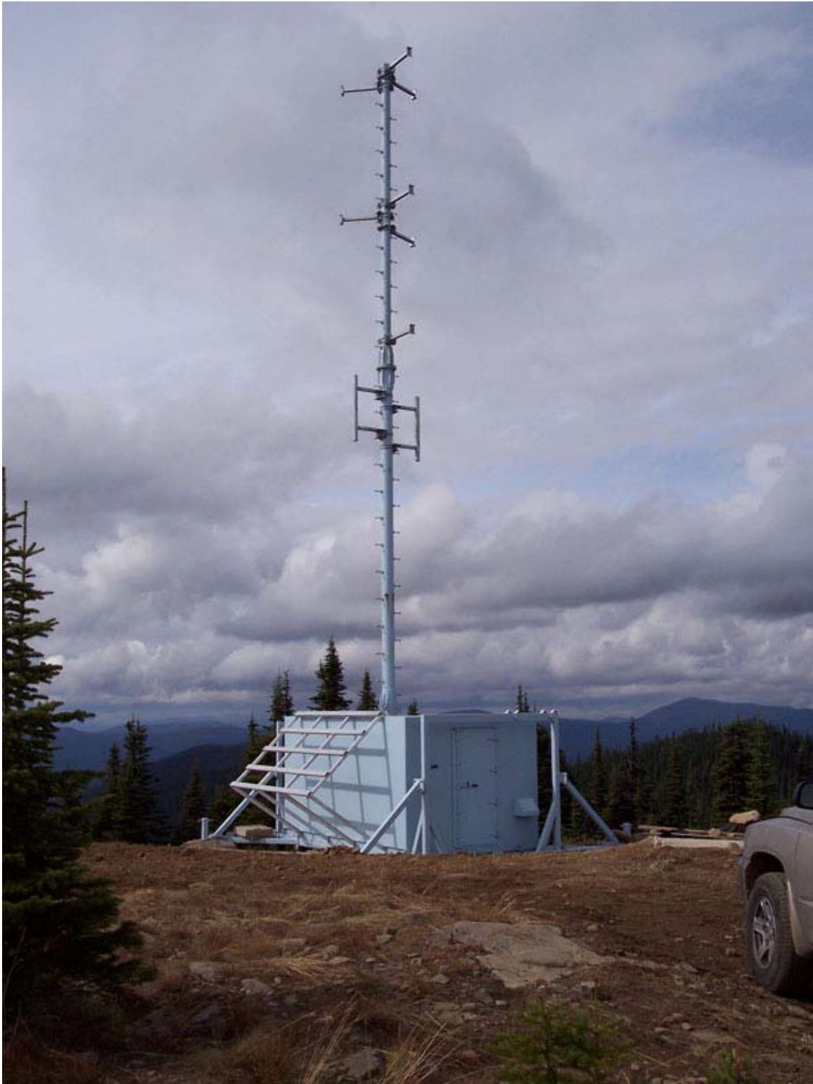
Example of a Shelter 8ft X 8ft X 8ft With Articulated Tower (approx. 40 ft)
