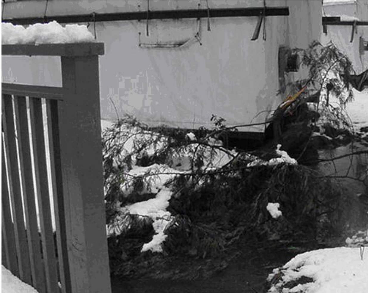
Photo 1 Drainage Channel Blocked by Tent #68, Making 90 Degree Bend to Left and Under Bridge
