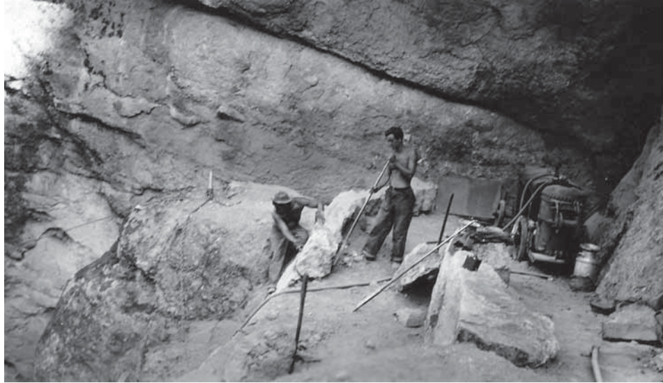
Figure 35. CCC enrollees positioning large boulders at switchback on High Peaks trail. [Narrative Reports, CCC Coll., RG 35, Box 22, NARA II.]
