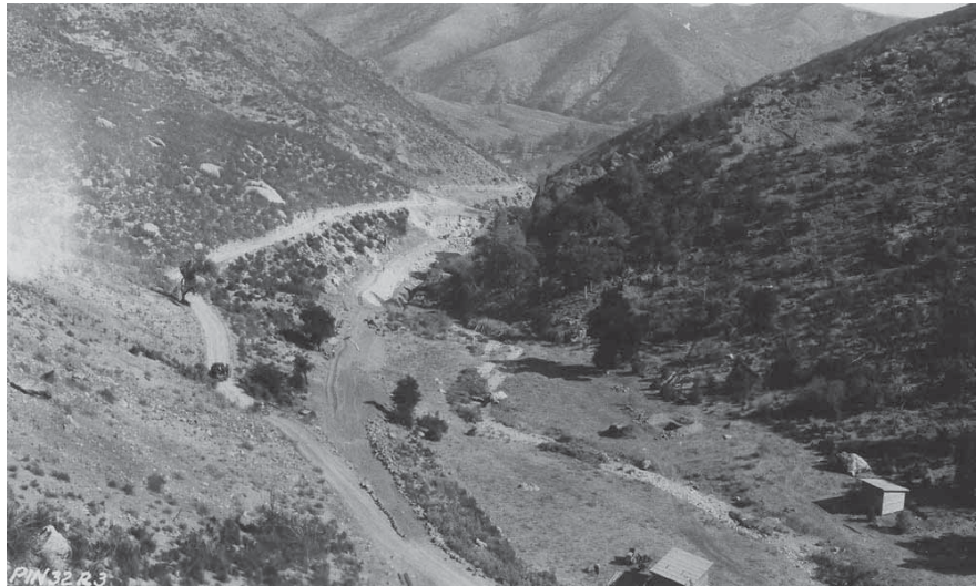
Figure 25. View from above looking east down Bear Gulch in early 1933. Original 1925 road is still extant to left. New road in progress below it. The buildings to the right are the blacksmith's shop and powder room. They were removed shortly after the project was completed. [Included in E.A. Kittredge, "Final Report on Construction of Entrance Road," April 15, 1933, Mus. Coll. PINN 3658, PNM.]
