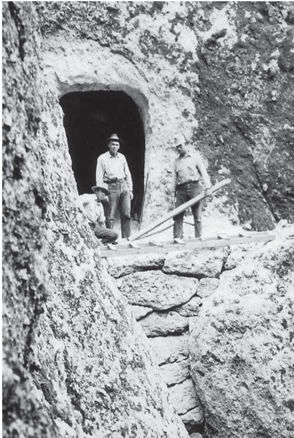
Figure 19. Local men working on High Peaks Trail, ca. 1932, with recently completed tunnel in background. The man standing in the middle of the group is probably crew boss Fred Prewett. [Mus. Coll. PINN 4372, PNM.]
