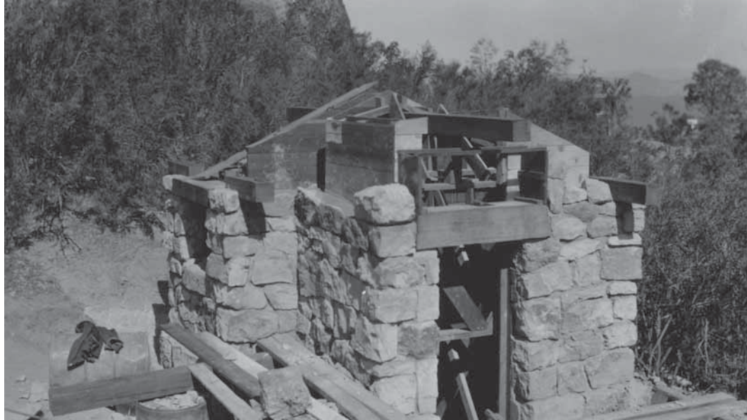
Figure 38. CCC enrollees in process of constructing rustic vault toilet at Scout Peak on the High Peaks trail. [Narrative Reports, CCC Coll., RG 35, Box 22, NARA II.]
