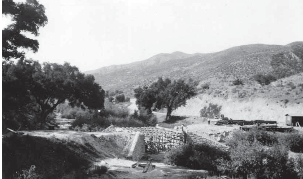
Figure 39. Construction of original Chalone Creek Bridge in spring of 1936. The stone abutments have been completed and the forms are being put in place to lay the deck. [Landscape Architects' Reports, PINN Coll. 3658, Misc. Boxes, PNM.]
