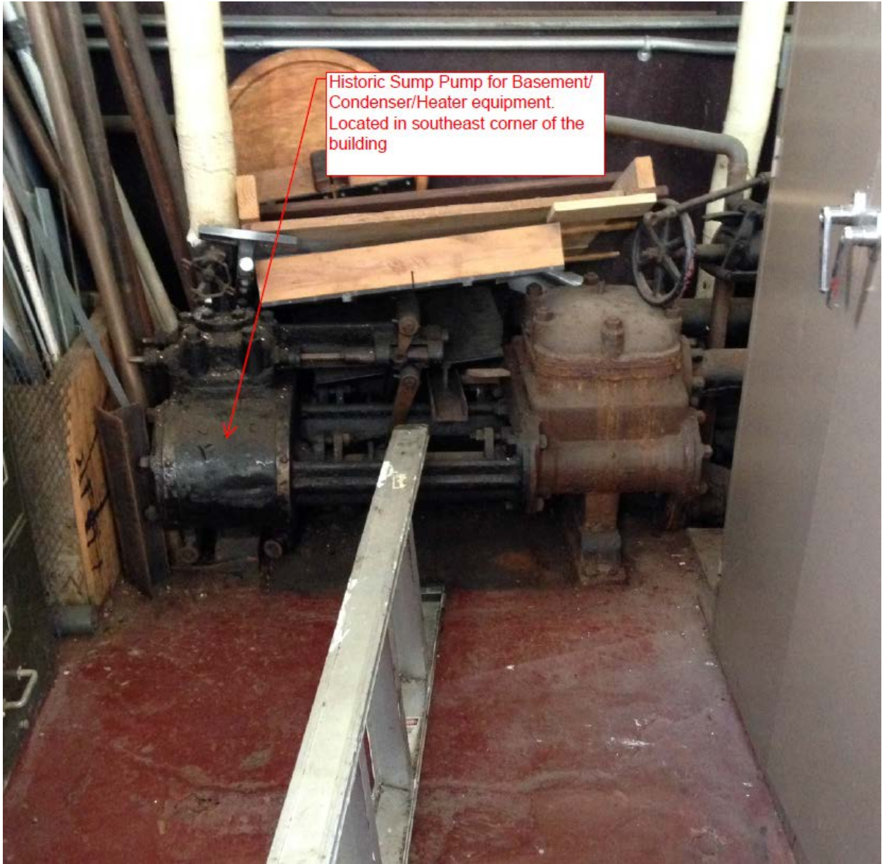
FIGURE 22 - Sump Pump in southeast corner of building.
