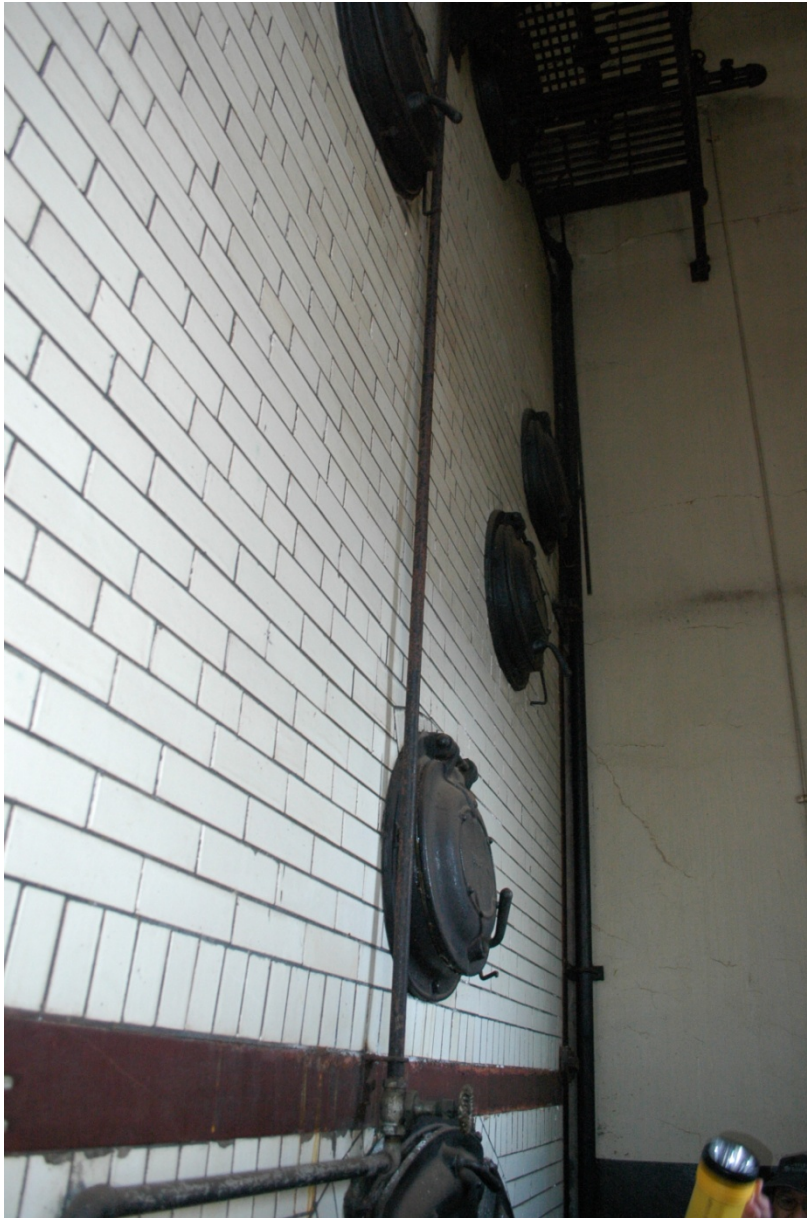
FIGURE 2 - Side of a boiler showing glazed tiles
