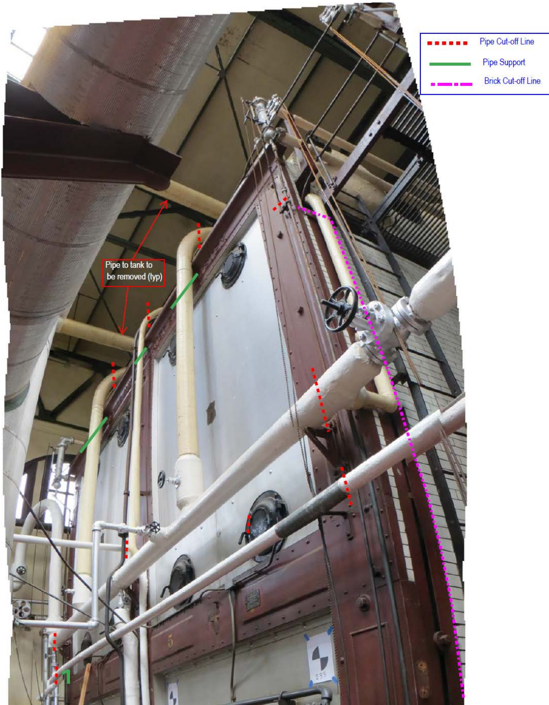
FIGURE 6 - Boiler façade, side.
