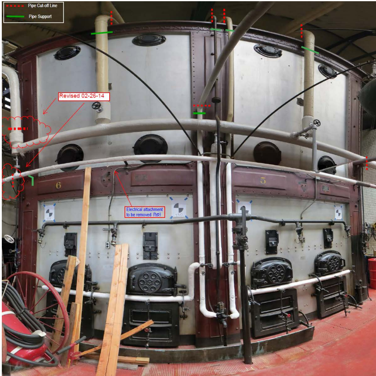
FIGURE 3 - Piping in front of a boiler (Boilers 5&6)
