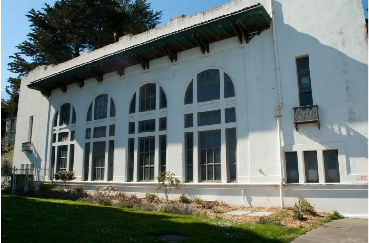
FIGURE 19 - Eastern side of Pump Station No. 2, showing windows to be replaced at the far right and left, and four sets of Bay windows (to remain) in the center.
