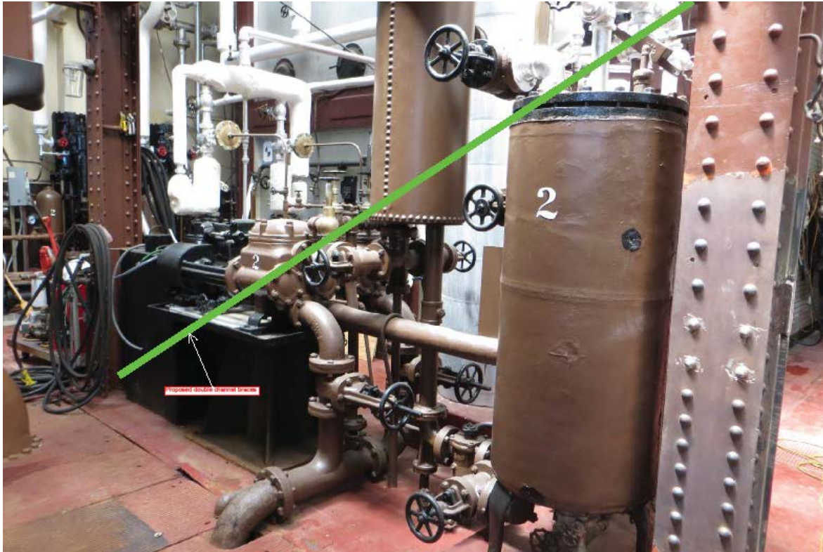
FIGURE 18 - Boiler feed pump. Location of proposed diagonal bracing is shown in green.
