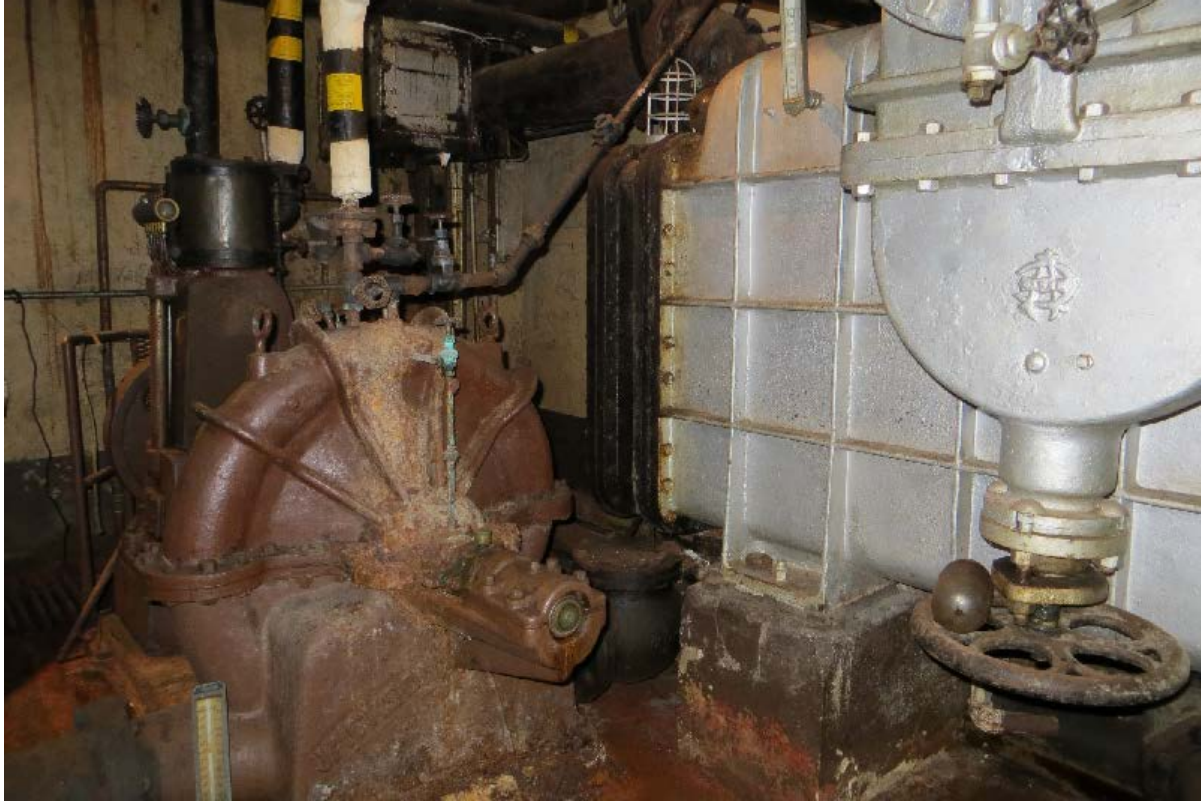
FIGURE 15 - Basement circuit pump (brown equipment at left) and condenser (silver equipment at right)
