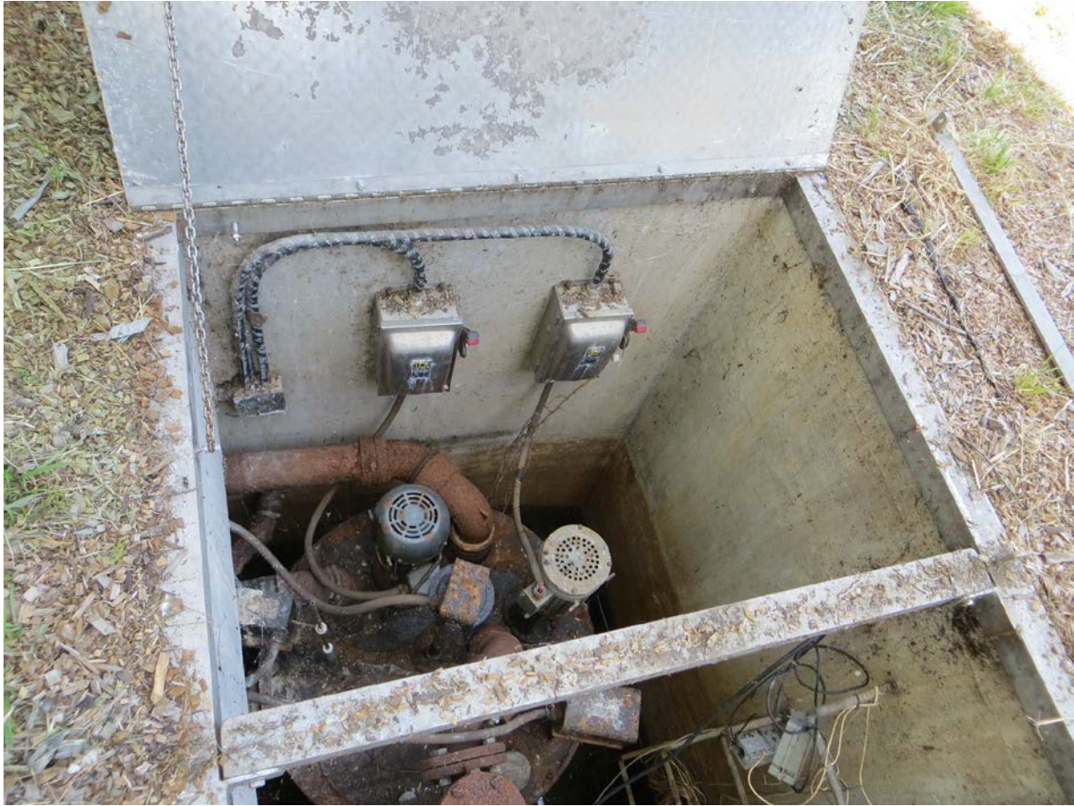
FIGURE 24 – Existing disconnect switches in a vault north of the building. New disconnect switches, to be mounted on the northern façade of the Pump Station (as seen in the next figure) would be similar to the existing switches.
