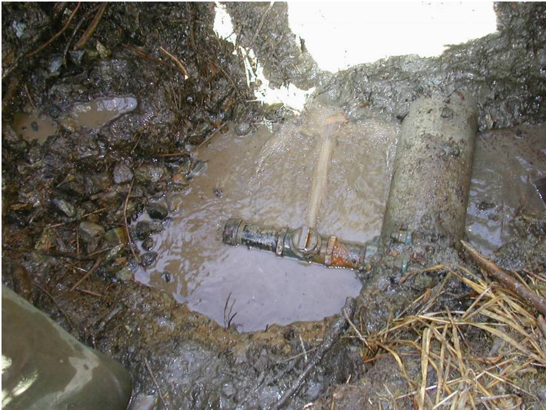
Photo 3 The Leak, before Repair
