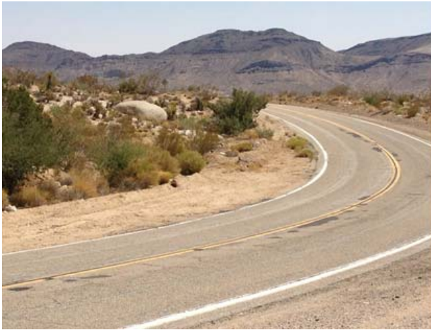
Photo showing sharp curve and abrupt grade change at Site 3
