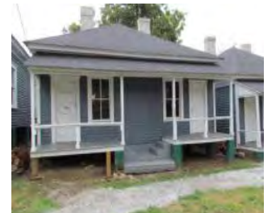
493 B Auburn Ave., one of three shotgun houses
