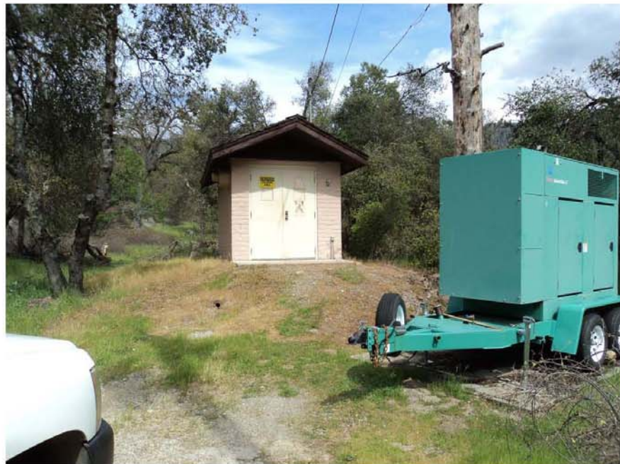
EP Well #3 House
