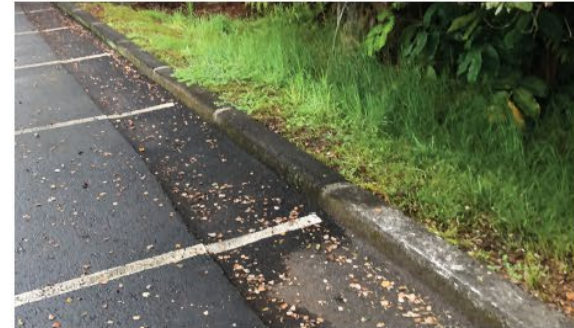
CURB - CONCRETE MATCH EXISTING CONCRETE CURB ON SITE IN TEXTURE, COLOR, AND USE OF SECTIONS WITH MORTAR JOINTS
