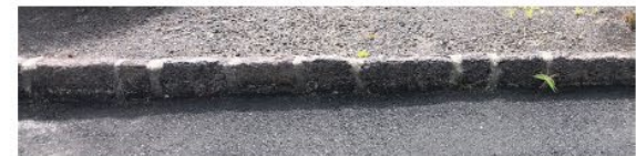
CURB - STONE CURB STONE WILL BE SALVAGED TO BE REUSED ON SITE
