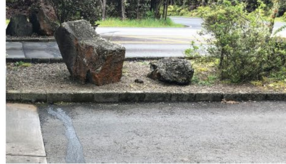
CURB - STONE CURB STONE WILL BE SALVAGED TO BE REUSED ON SITE
