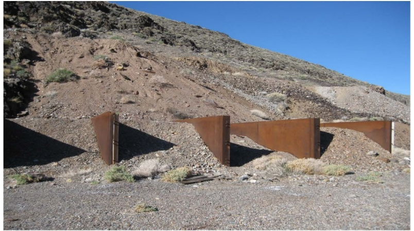
Figure 1 - View of cyanide processing area and crushed ore used for mill foundation looking south.
