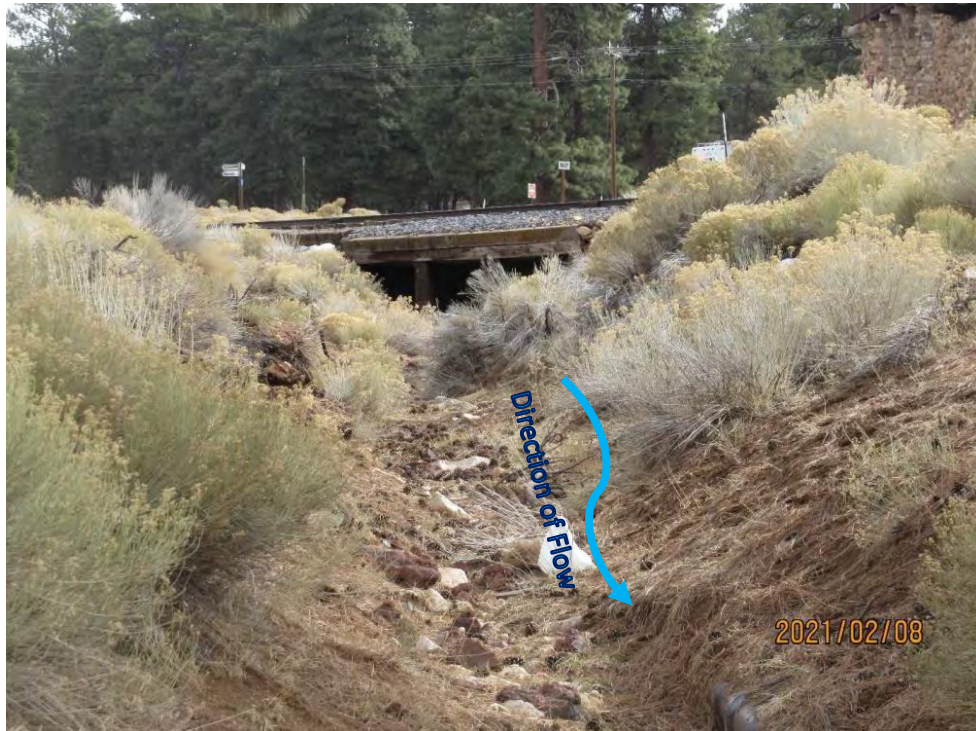
View east showing Bright Angel Wash and the railroad crossing proposed for replacement. The Powerhouse building is visible on the right side of the photo (January 8, 2021).
