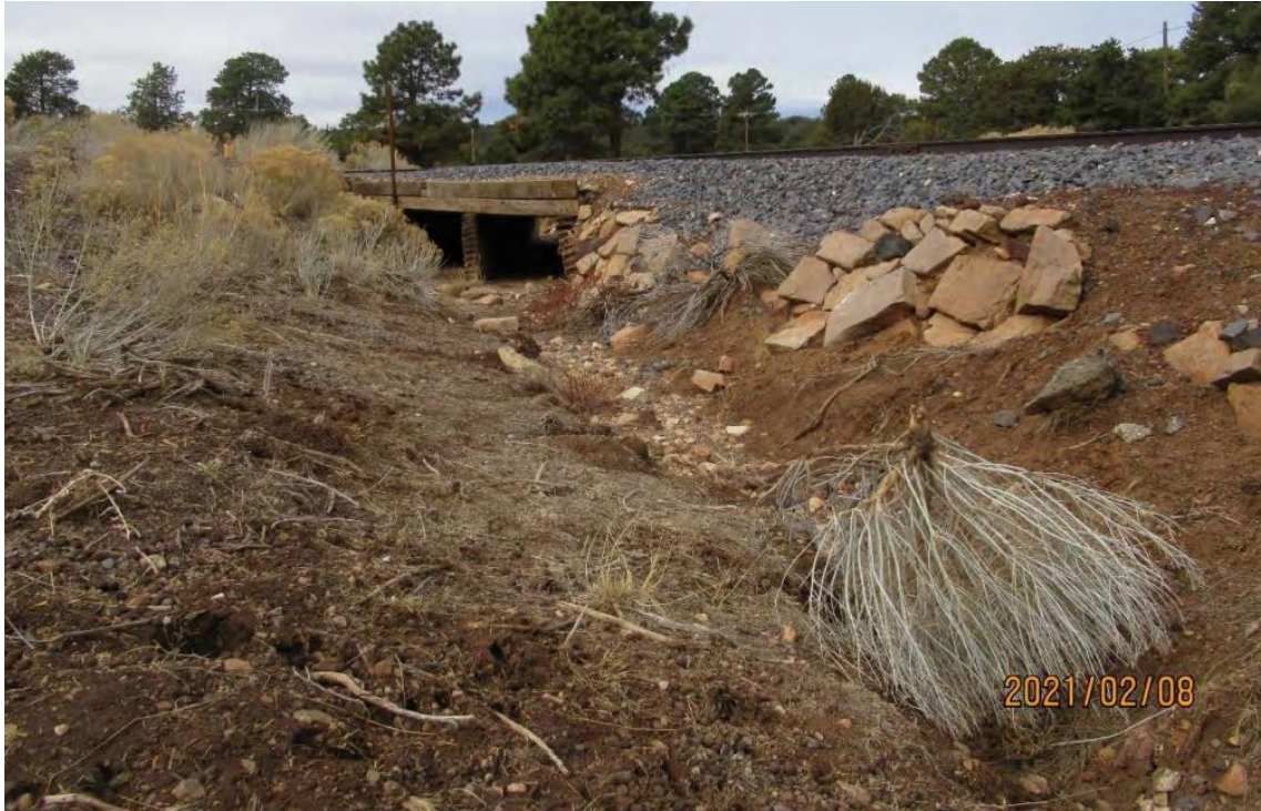
View west showing Bright Angel Wash and the railroad crossing proposed for replacement (January 8, 2021).
