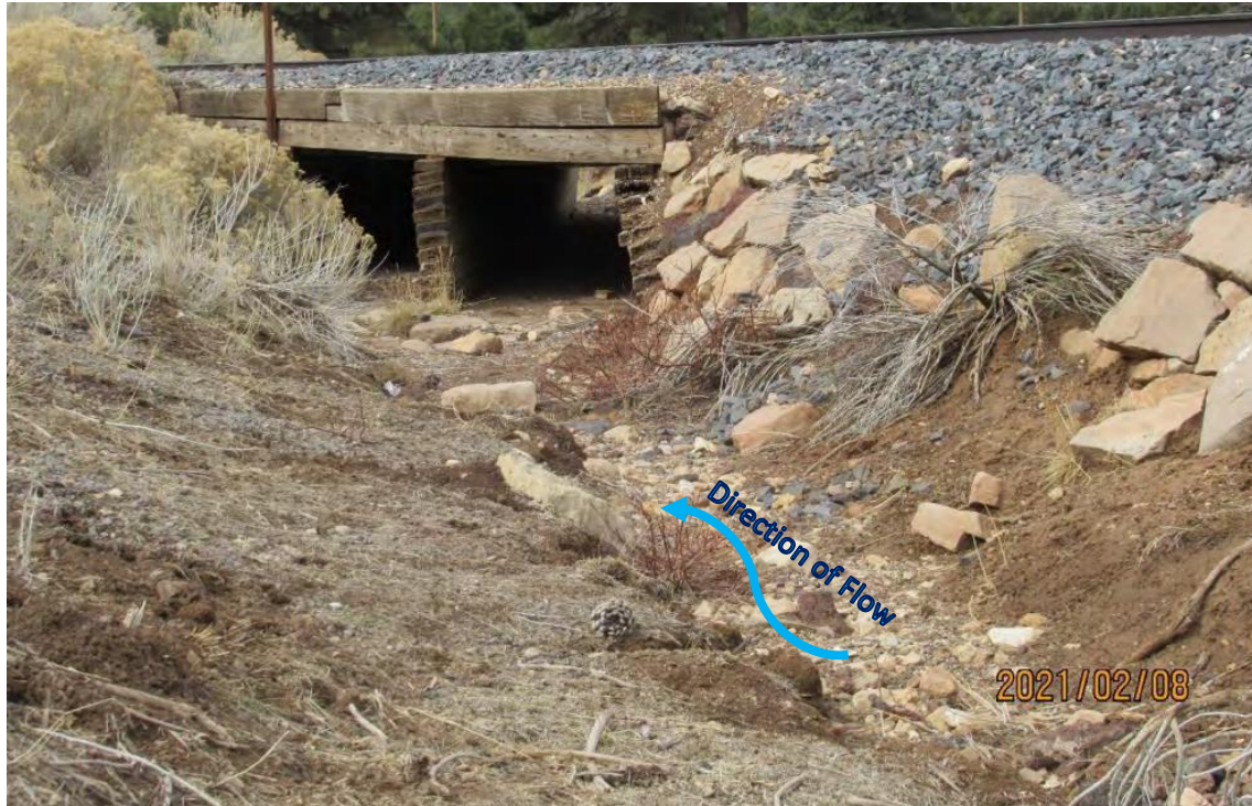
View west showing Bright Angel Wash and the railroad crossing proposed for replacement (January 8, 2021).
