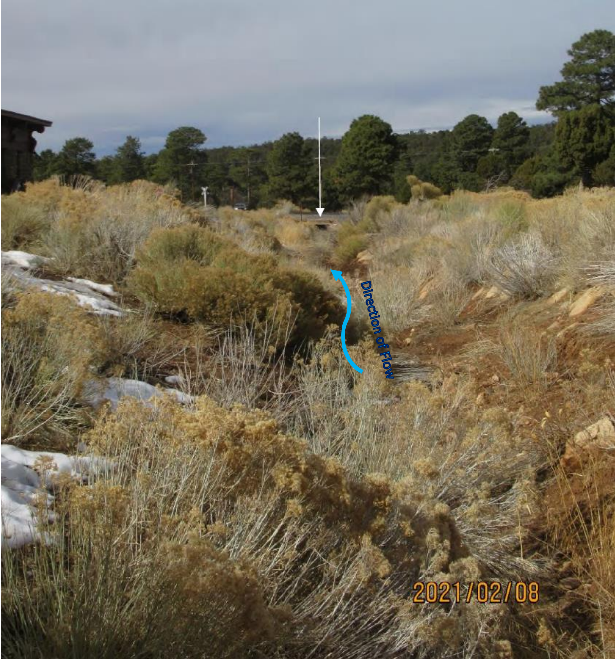
View west showing Bright Angel Wash and wooden box culvert (white arrow).
