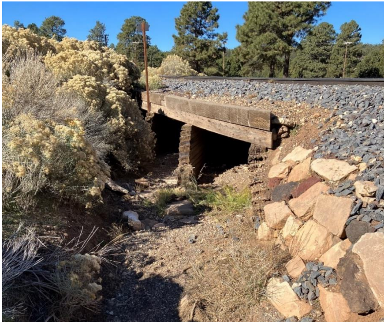
Bright Angel Wash on the east side of the wooden ballast bridge, looking west (11/7/22)
