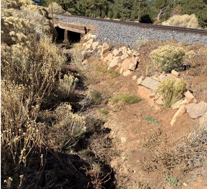
Bright Angel Wash on the east side of the wooden ballast bridge & drainage, looking west (11/7/22)
