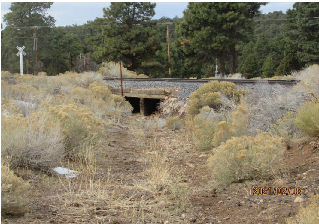
View west showing Bright Angel Wash and the railroad crossing proposed for replacement (January 8, 2021).
