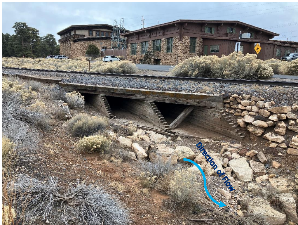
Bright Angel Wash on the west side of wooden box culvert, looking southeast (January 3, 2024)
