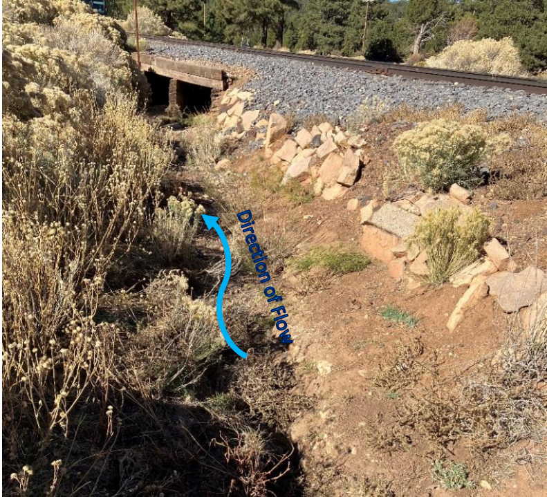
Bright Angel Wash on the east side of the wooden box culvert, looking west (11/7/22)
