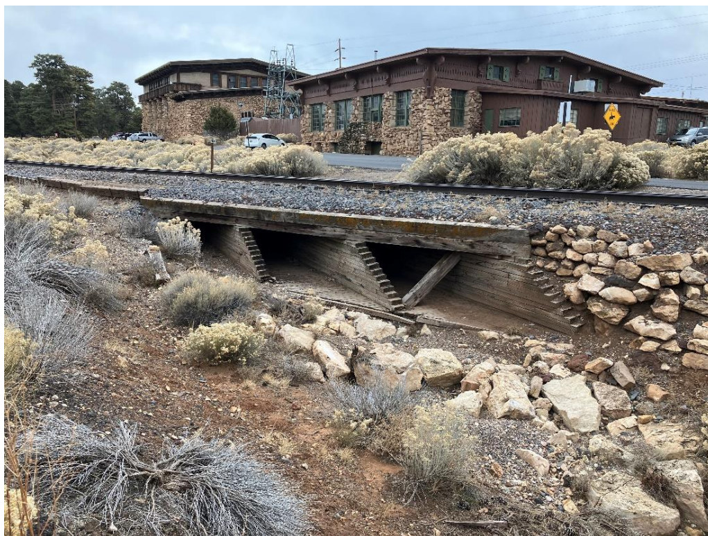
Bright Angel Wash on the west side of wooden ballast bridge, looking southeast (January 3, 2024)
