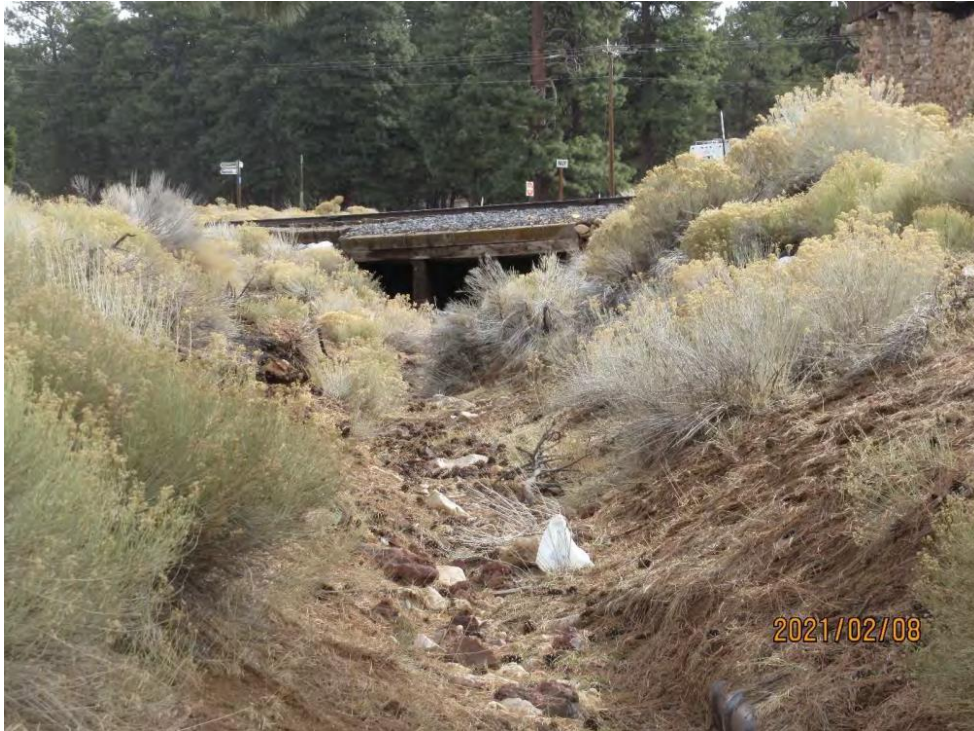
View east showing Bright Angel Wash and the railroad crossing proposed for replacement. The Powerhouse building is visible on the right side of the photo (January 8, 2021).
