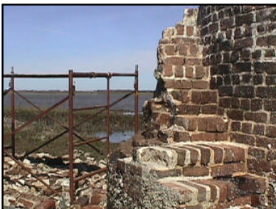
Damaged lighthouse steps.
