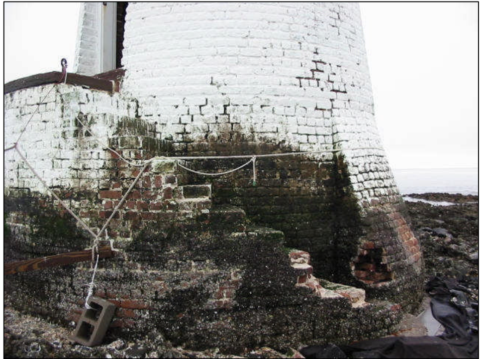
The NPS has been making emergency repairs to the lighthouse's exposed wooden foundation that is being damaged by shipworms.
