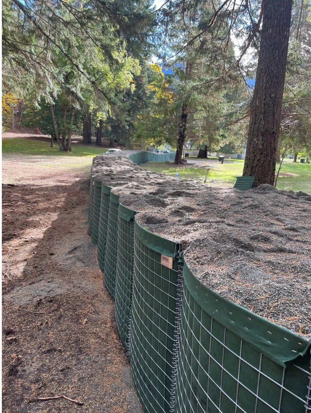
Figure 6. Example of HESCO barriers
