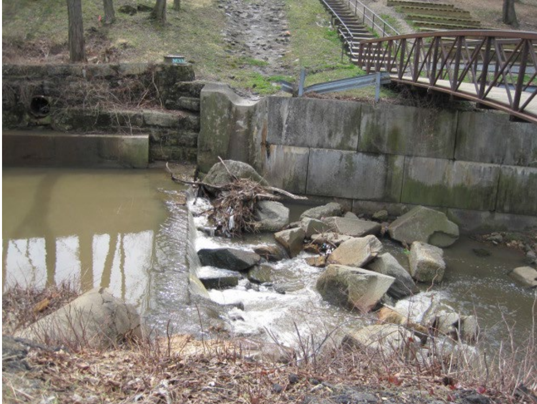
Sewer Infrastructure in Stream- Before
