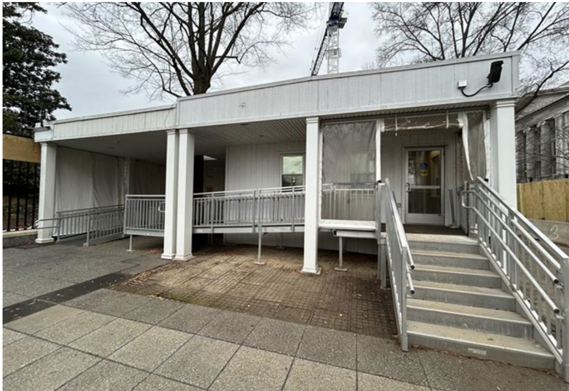
VIEW OF THE EXISTING VISITOR SCREENING TRAILER ENTRANCE ON EAST EXECUTIVE AVENUE.
