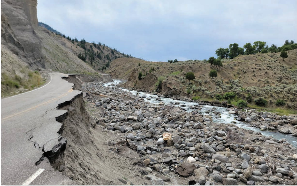
GAMA001s_135_pp – Road damage along Gardner River (GAMA001s). View is to the southeast.
