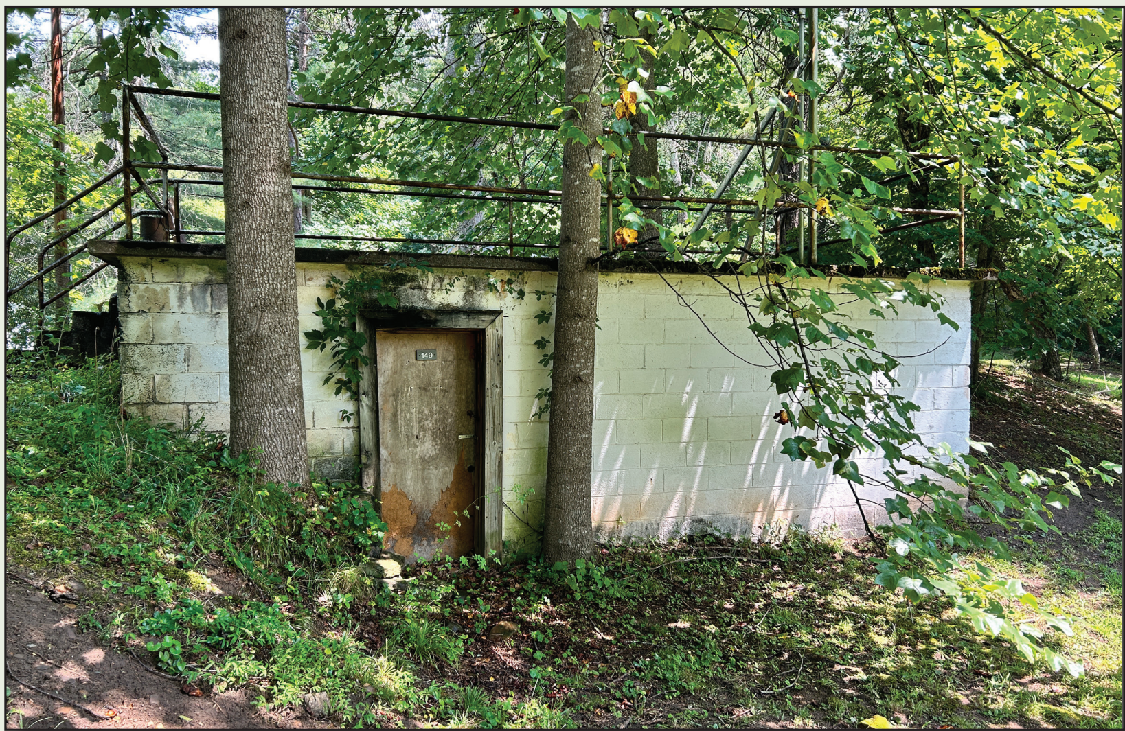
19 Camp Brookside Pool Chemical Treatment Building
