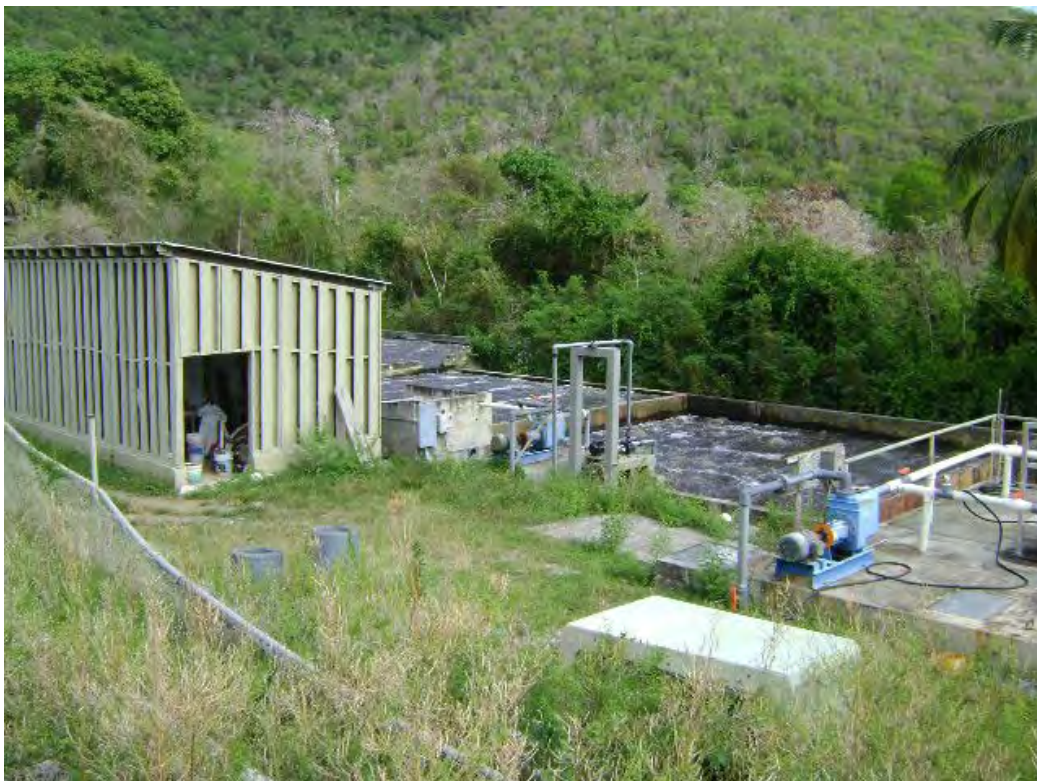
Wastewater Treatment Plant Area
