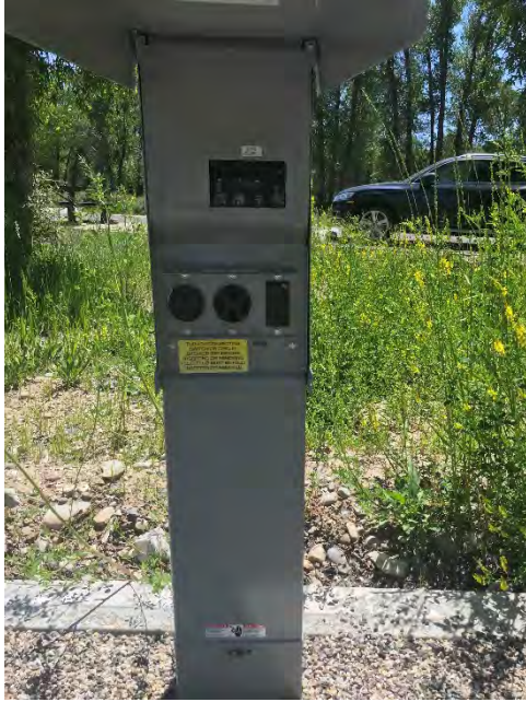
Figure 3.82 Electrical camp site panel with 30-amp and 50-amp connections. Consider locking bottom portion of panel to prevent tampering with electrical capacity.
