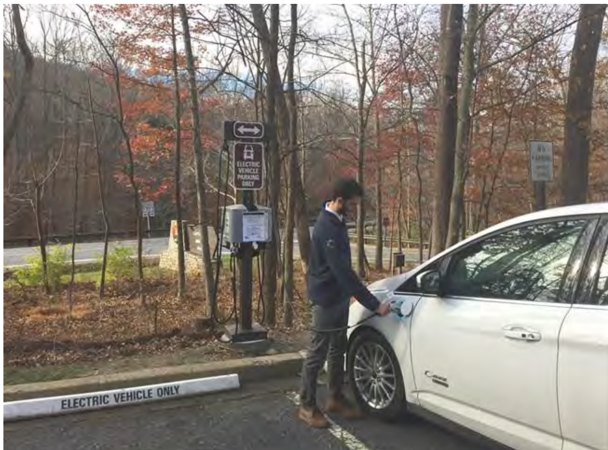
Figure 3.109 Example of Electrical vehicle charger installed at Catocin Mountain Park, Maryland. Charger installation requires a transformer that can accommodate the charging stations. This may require a new transformer, new panel, new disconnect switch, meters, bollards, electric vehicle parking signs and striping, electrical conduits, and the charging stations themselves.
