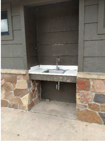
Figure 3.81 The outdoor dish washing sinks at Glacier Basin campground in Rocky Mountain National Park are integrated on the comfort station exteriors and provide a firm and stable surface and knee clearance for accessibility.
