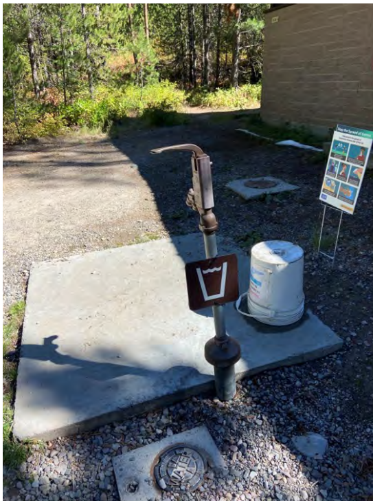
Figure 3.65 Grand Teton National Park, Wyoming, Signal Mountain Campground, accessible frostproof water hydrant that can be operated with a closed fist.
