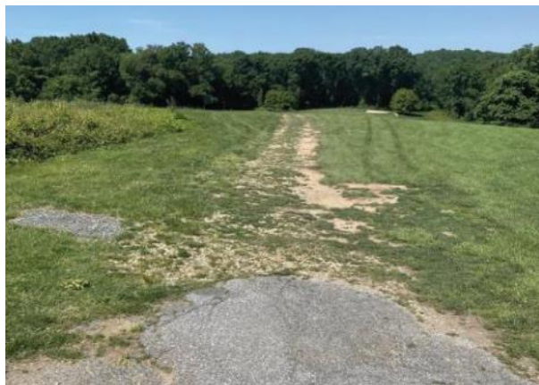
View of deteriorated asphalt and worn grass cart path
