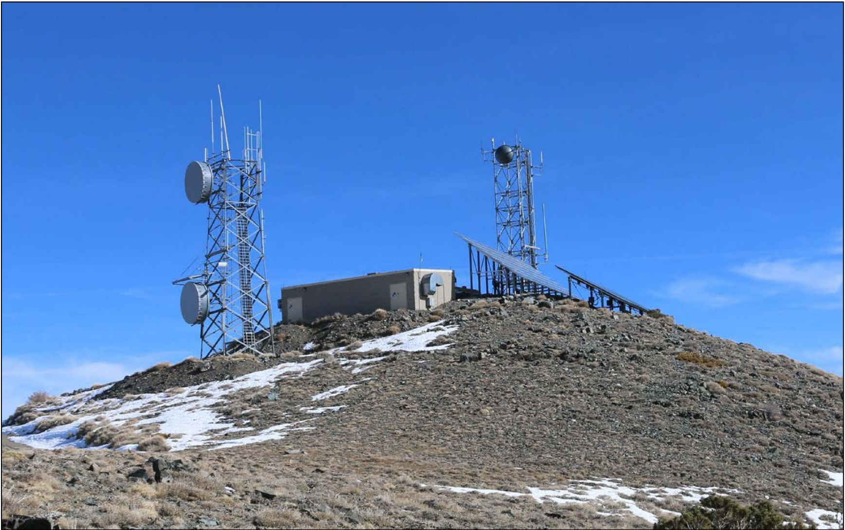
FROM LEFT TO RIGHT: CALTRANS TOWER, CALTRANS COMMUNICATIONS BUILDING, US AIR FORCE SOLAR PHOTOVOLTAIC ARRAY, US AIR FORCE TOWER, SOUTHERN CALIFORNIA EDISON SOLAR PHOTOVOLTAIC ARRAY
