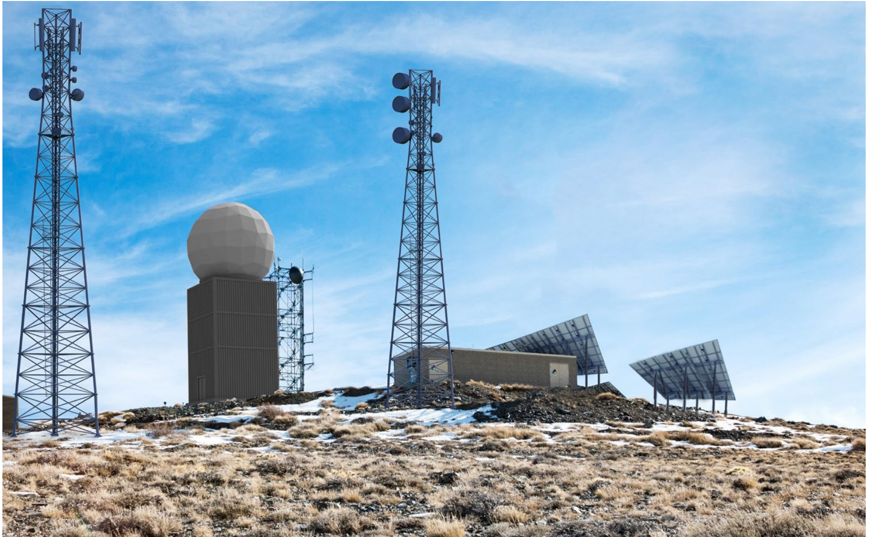
FROM LEFT TO RIGHT: PROPOSED AT&T COMMUNICATIONS BUILDING, AT&T TOWER, US NAVY RADOME, US AIR FORCE TOWER, CALTRANS TOWER, CALTRANS COMMUNICATIONS BUILDING, SOLAR PHOTOVOLTAIC ARRAYS
